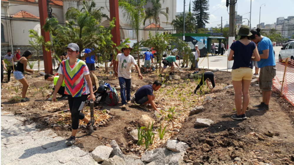
Figure 11. Community planting, 16.12.2017, the first rain garden in a Brazilian city, in a central area in São Paulo. A learn-by-doing experience. (Brazilian Case Study 13).
